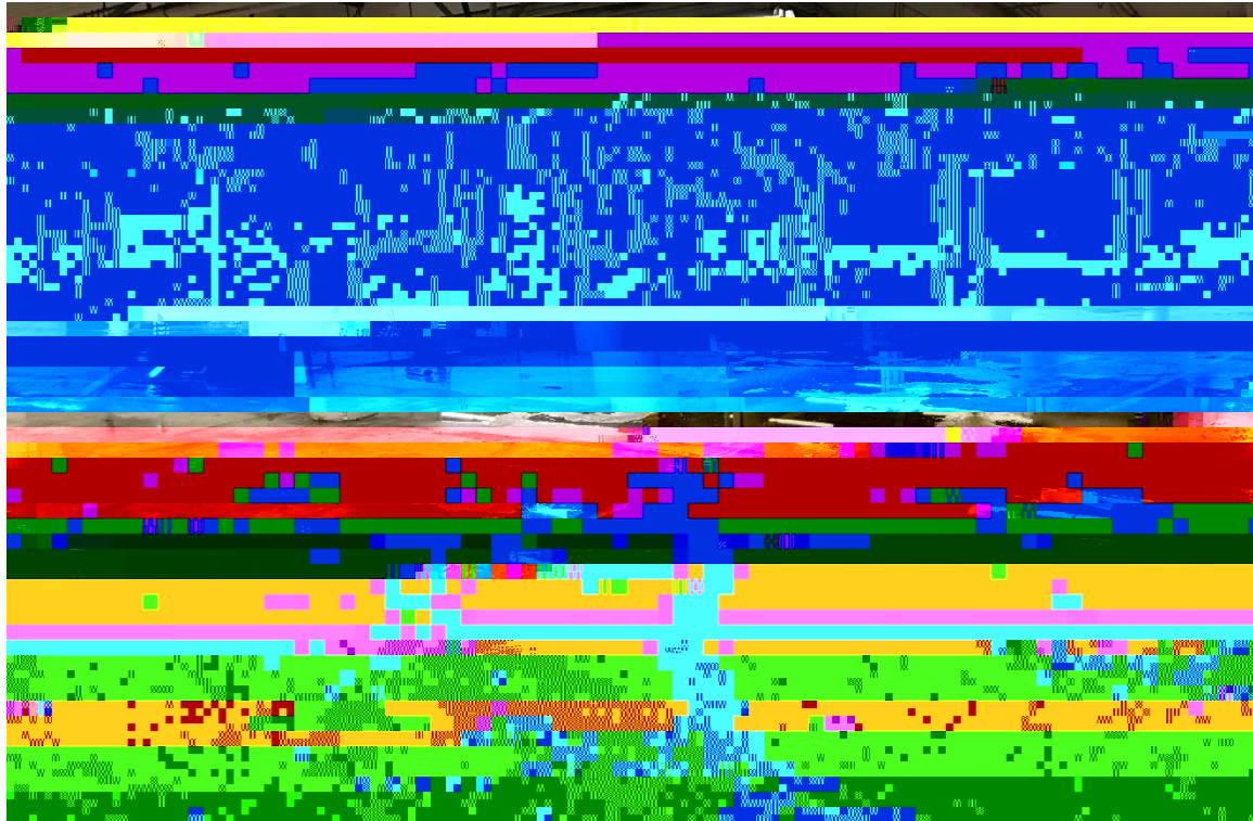
Flooding in northern portion of Building C basement
