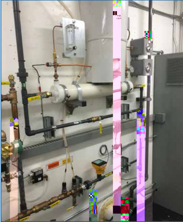
Groundwater injection system components.
