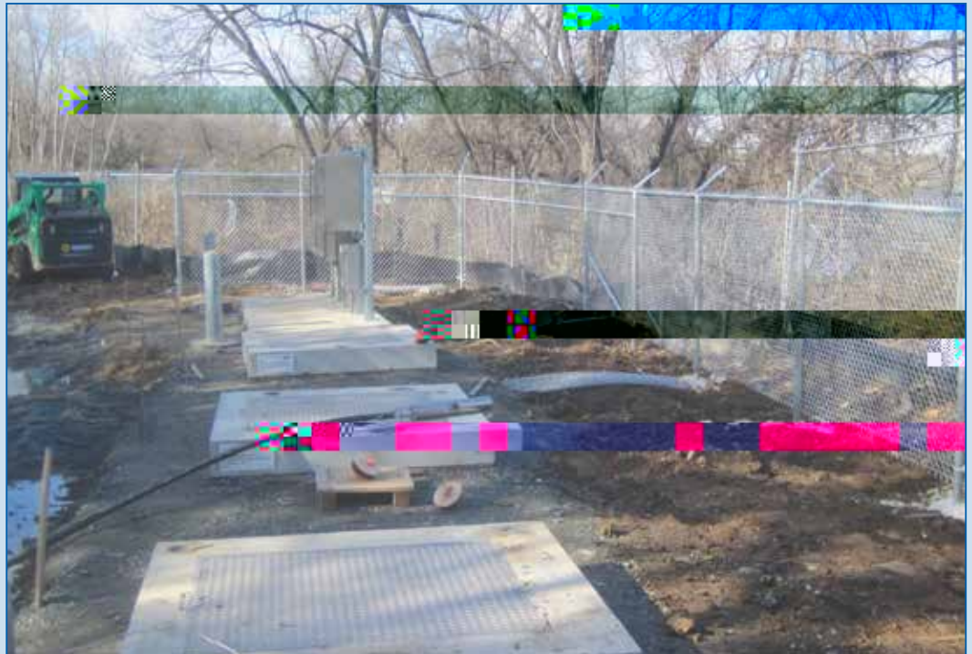
Fencing surrounds the site, including extraction wells, and includes a locked gate allowing access to the outfall pipe on Frog Mortar Creek.
