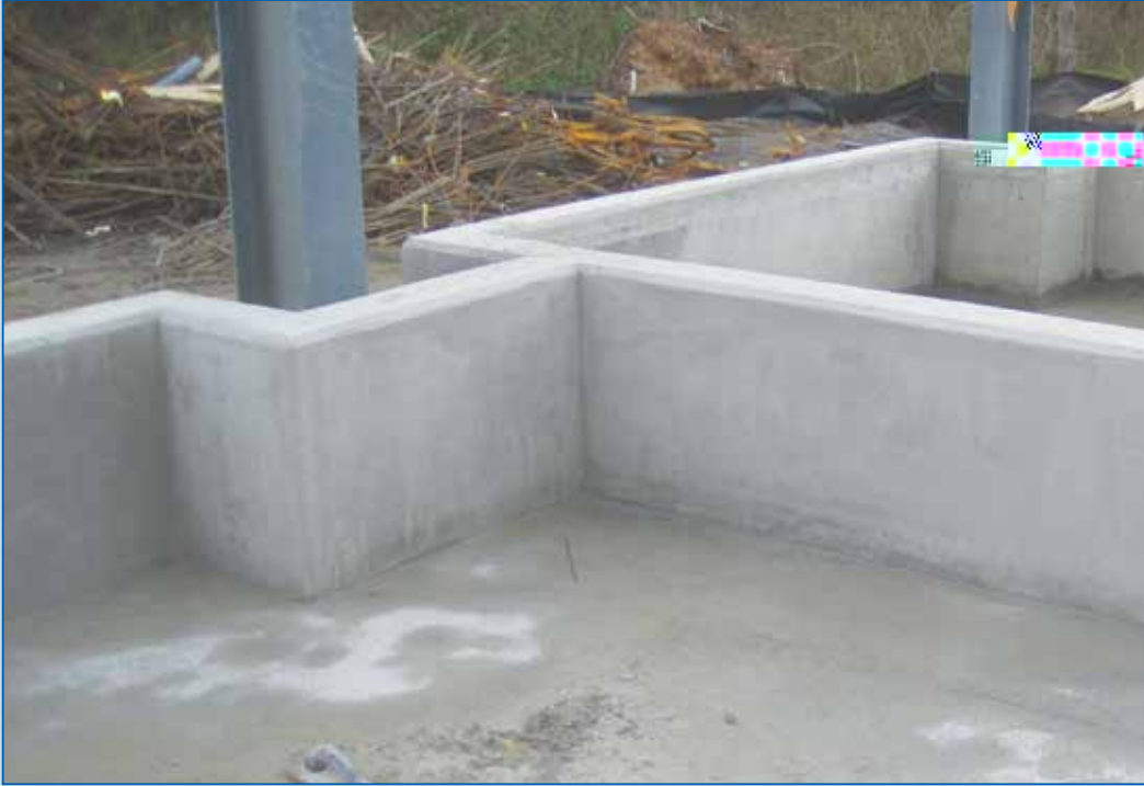
A hardener and sealant were applied to finish concrete floors and containment walls.
